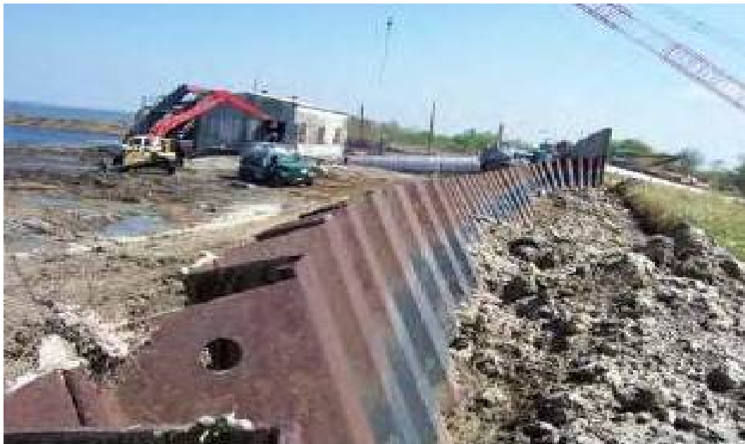
Figure 1. Damaged Section of Levee after Hurricane Katrina (LPV-111)
