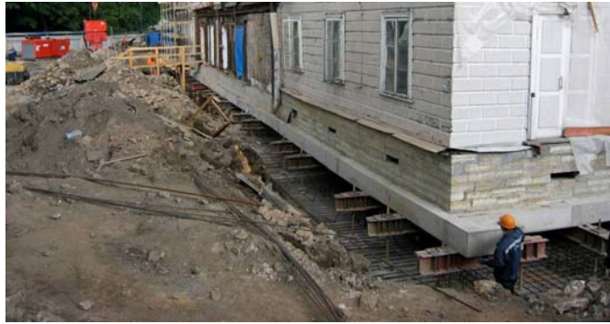
Figure 3. Suspension of the building on Titan piles to provide construction of the rigid disc slab
