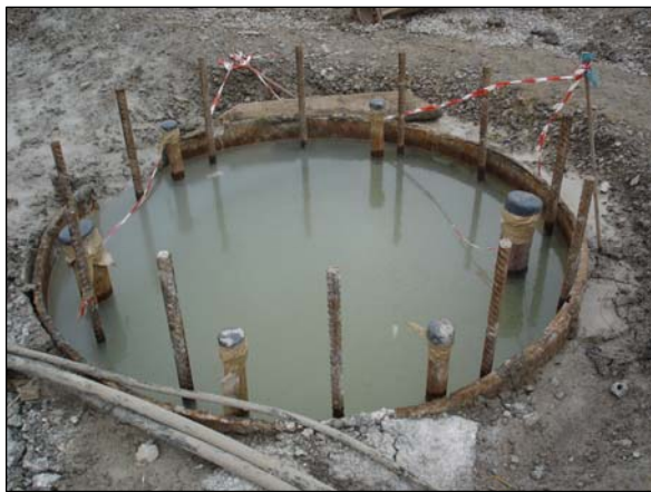
Figure 7. Pipes set up for shaft control
