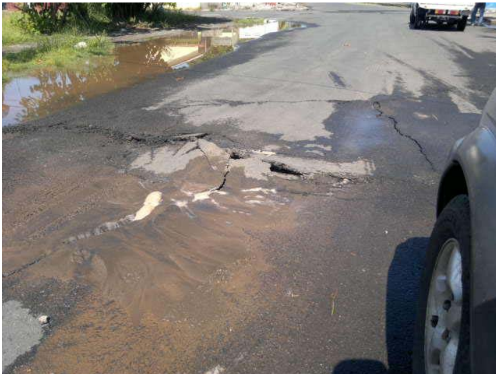
Fig. 7 Sand boiling through a cracked pavement in Puntarenas.
