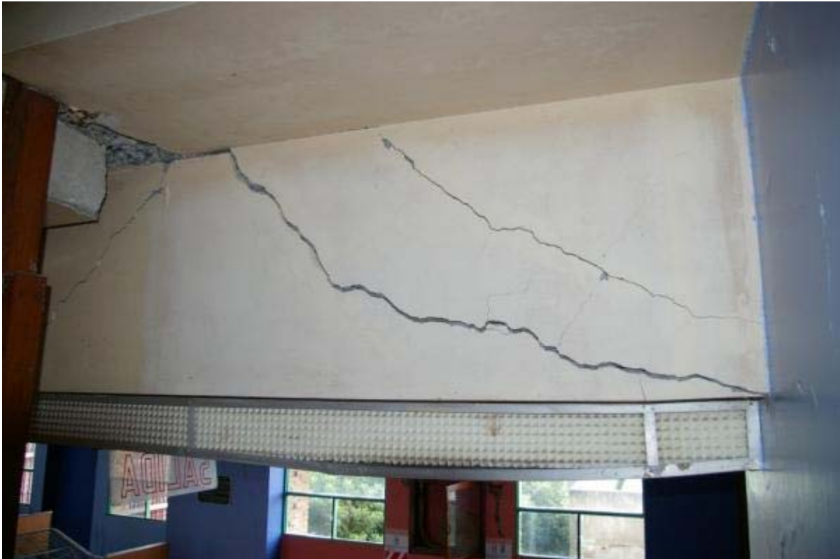
Fig. 11 Shear cracks in the floor beams of the main stairs of the Hospital Monsenor Sanabria. Source: Laboratorio de Ingenieria Sismica, Universidad de Costa Rica.
