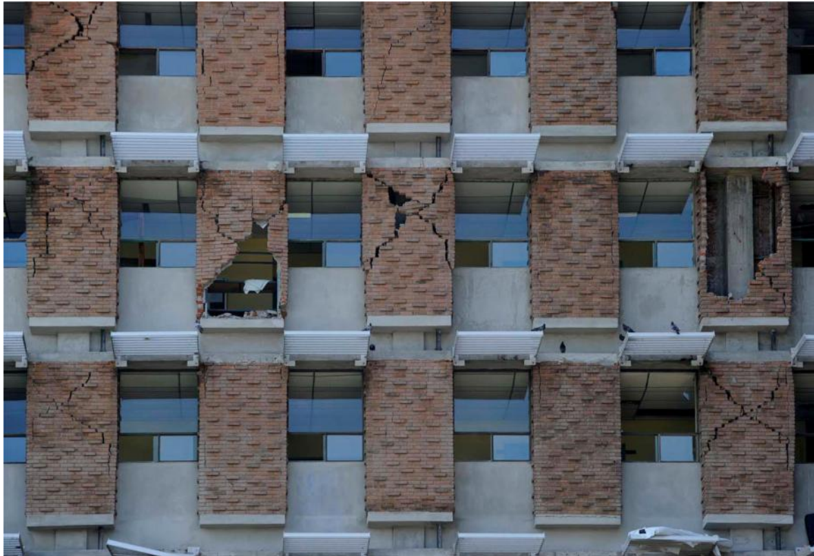
Fig. 10 Shear failure of non structural facade walls of the Monsenor Sanabria Hospital (Source: La Nacion, online version).
