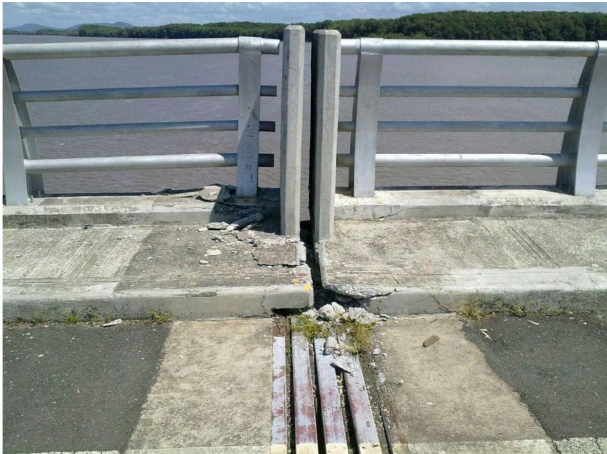
Fig. 9 Collision and permanent relative displacement between the two spans of the Amistad bridge (Source: La Nacion, online version).
