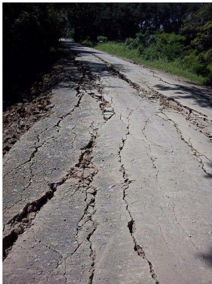
Fig. 8 Tension cracking and slope failure of the Tempisque levee at Filadelfia (Source: La Nacion, online version).
