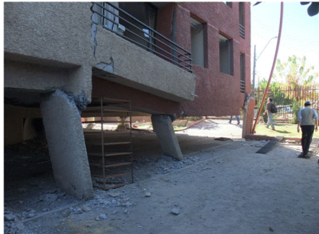
Photo 28 Collapsed building at Maipú in Santiago
