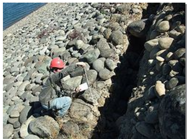
Photo 10 Downward slope movement in upstream face
