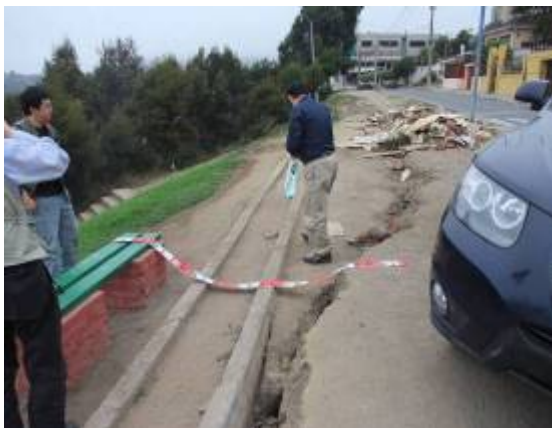
Photo 13 Minor slope failure at San Antonio
