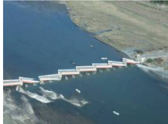
Photo 15 Collapsed bridge in Tubul
