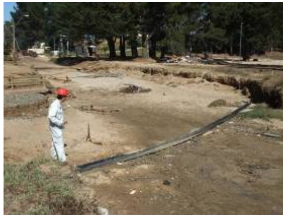
Photo 24 Exposure of buried lifeline after tsunami erosion
