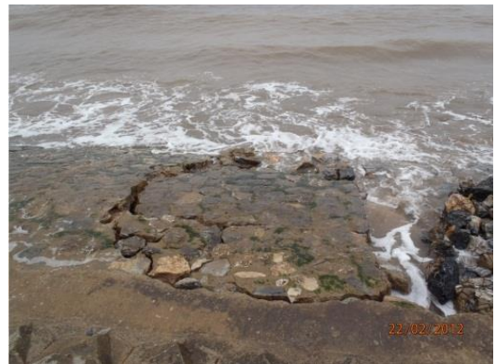
b) Destruction of inner slope by overtopping, Thinh Long 4 Dec 2013
