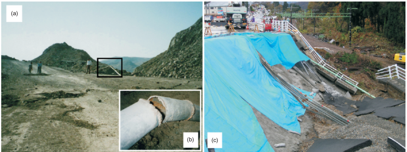
Fig. 1. Fault-induced damage of embedded pipeline during 1990 Manjil earthquake, Iran: (a) view of damage from a distance; (b) close-up of pipeline failure. (c) Damage to buried pipes embedded in an embankment along Highway 17, Kawaguchi, during 2004 Niigata-ken Chuetsu earthquake, Japan (37·291°N, 138·836°E)
