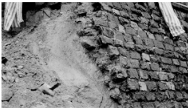
Fig. 14 Close view of the collapsed retaining wall
