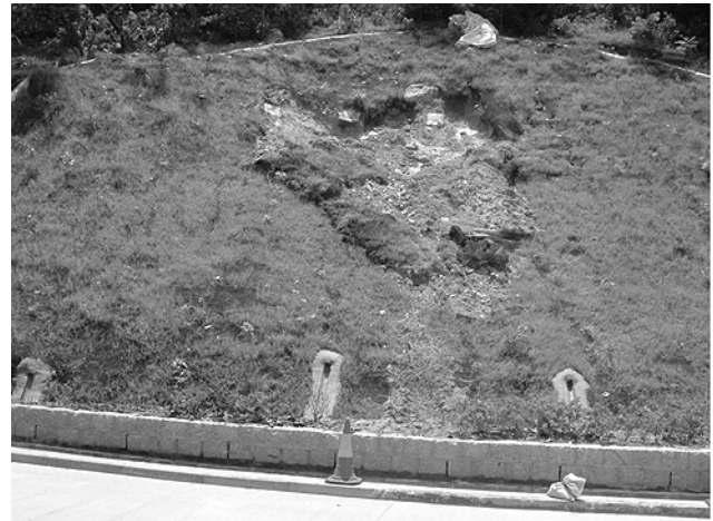
Fig. 22 Local failure at a soil-nailed slope
