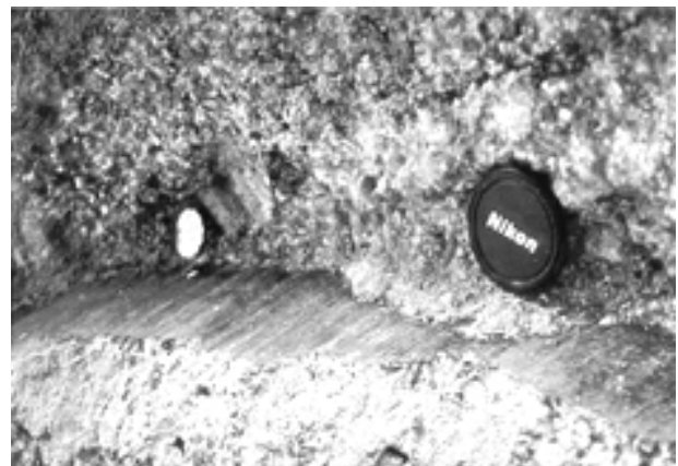
Fig. 20 Slickensided relict joint exposed at the 1999 Shek Kip Mei landslide
