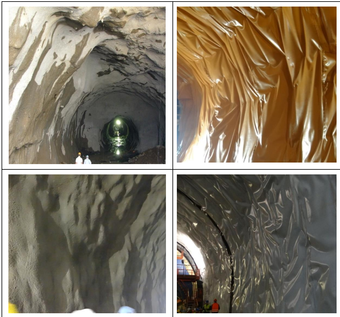
Figure 3 Only one of these photographs can be considered as 'unrepresentative' of the norm, and is clearly the too-shallow metro station (top-left) which shows overbreak as much as 4 meters. In fact it is photographed in the pre-concreting / post-shotcreting stage of the J_n/J_r > 6 , photograph in Figure 2. The other photograph of overbreak (bottom left) shows 'normal overbreak' which was (insufficiently?) shotcreted in a Norwegian tunnel, and where the white membrane (lower-right) is about to be applied. The yellow membrane (top-right) is from a metro tunnel in Hong Kong. In both membrane photos, a degree of 3D adjustment is evident, allowing the concrete to increase to at least 1 m thickness, instead of the minimum 35 cm as designed.
