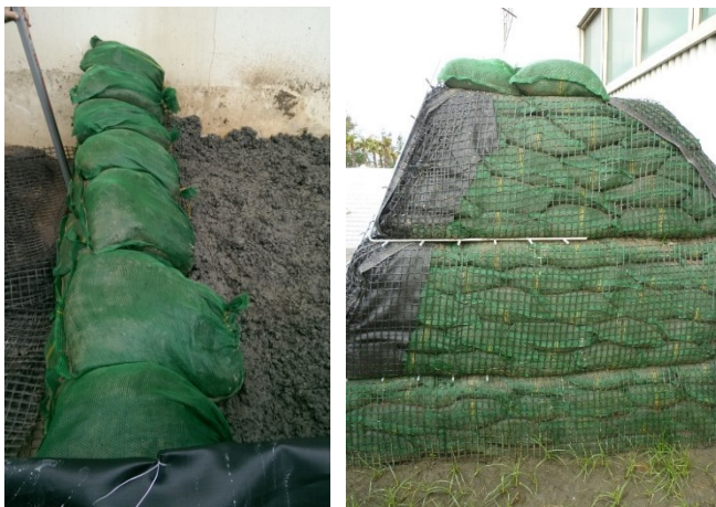
(a) Vegetation bags and CLSM (on the right) (b) Completed wrap-faced embankment
