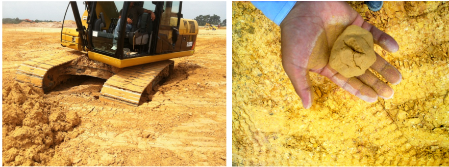
Figure 11 Uncompacted heavy silty clay
