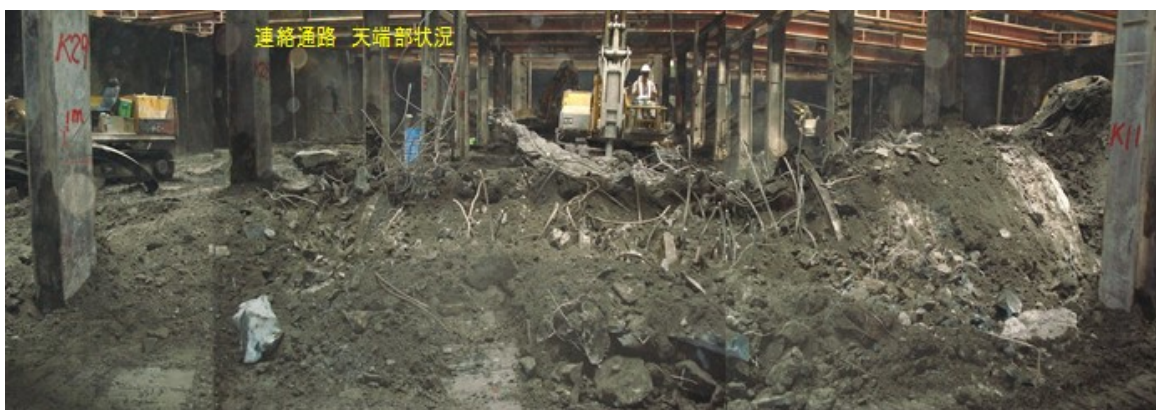
Figure 26 Wreckages of the crosspassage.
