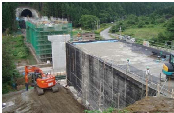
Fig.3 Geosynthetic Reinforced Soil Structure (GRS) in High Speed Rail (Tatsuoka et al , 2014)
