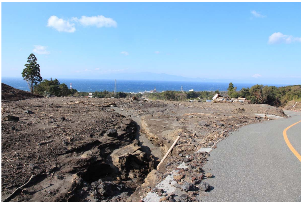
Fig. 6 Destroyed part of Moto-machi Town at the base of the slope
