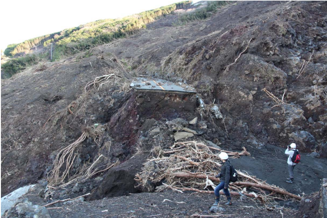
Fig. 5 Significant erosion in the middle part of the slope (see road pavement at the center and lava outcrop above the person on the right)
