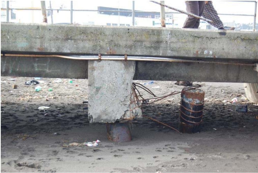
Fig. 17.- Evidence of the lateral displacements experienced by the liquefied ground
