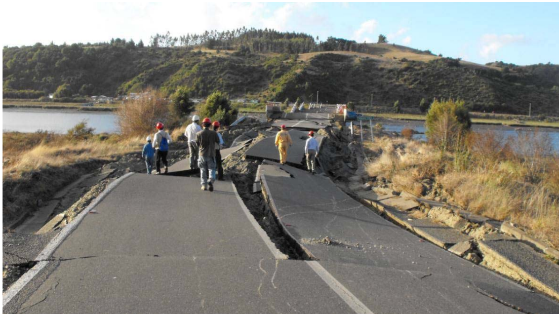
Fig. 6.- Failure of the access at bridge Tubul
