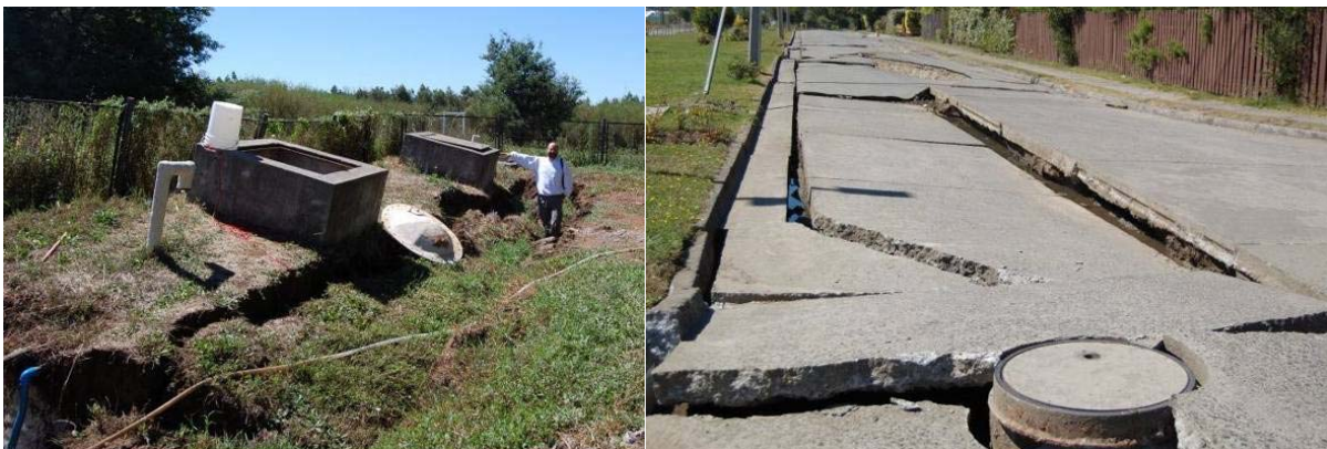
Fig.- 21.- Uplift of buried structures (Chillán and Arauco)
