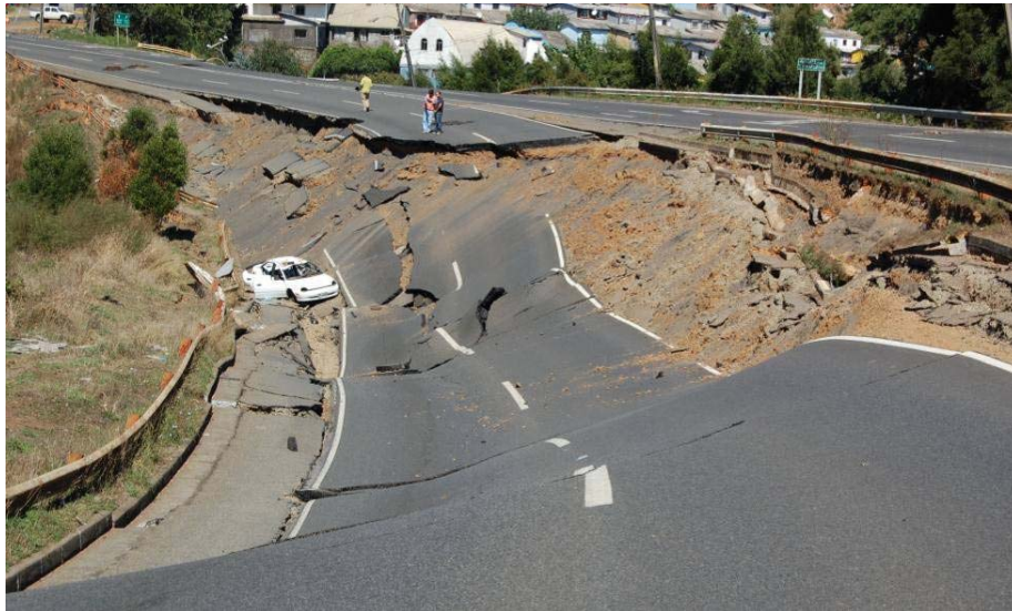
Fig. 5.- Failure of a fill triggered by foundation failure, Sector Polvorín, Ruta P160
