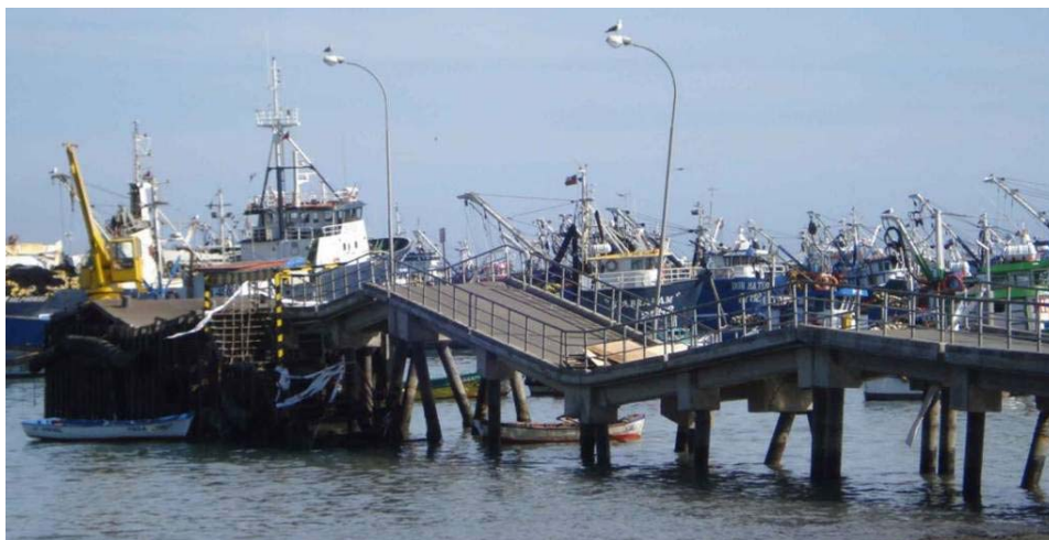
Fig. 16.- Large displacements experienced by a pier of local fishers
