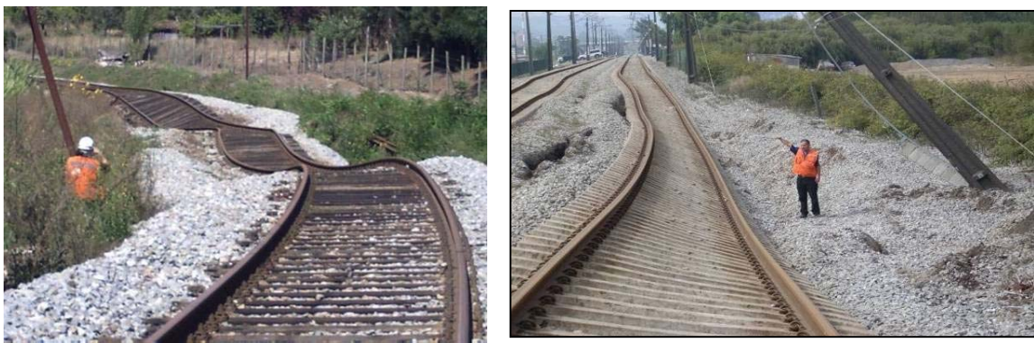
Fig. 10.- Settlements after liquefaction, near city of Concepcion (courtesy of EFE)
