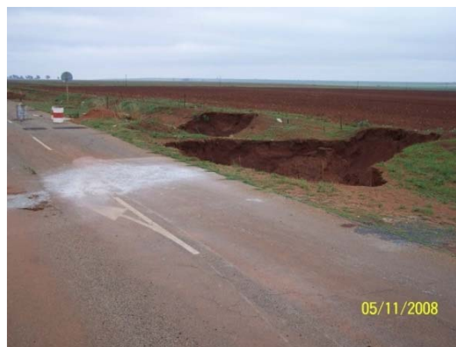
The two sinkholes that formed on either side of the culvert: Preliminary work
