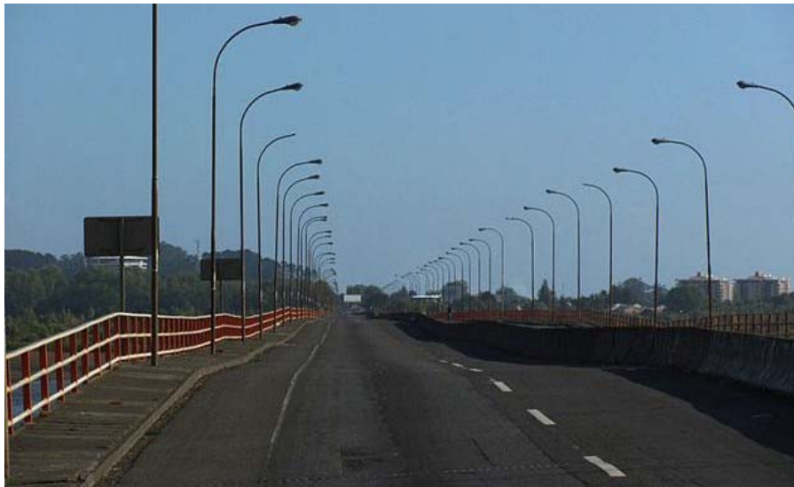
Fig. 13.- Differential settlements observed along Juan Pablo II Bridge, Concepcion
