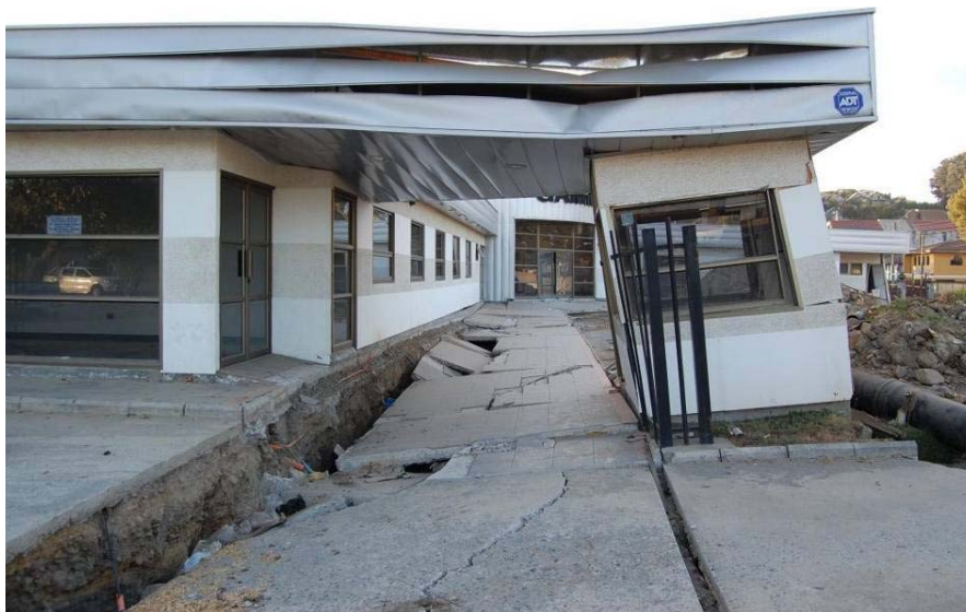
Fig. 14.- Failure observed in Constitucion city
