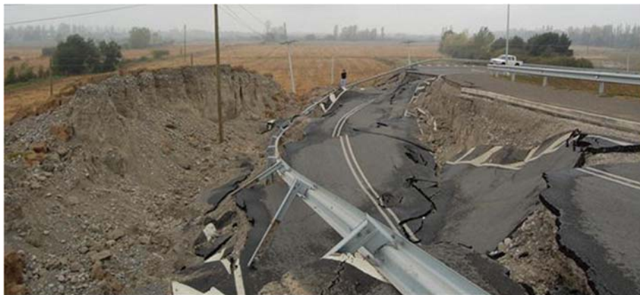
Fig. 3.- Failure of a fill triggered by foundation failure. Cruce Villaseca, Km37-Ruta5
