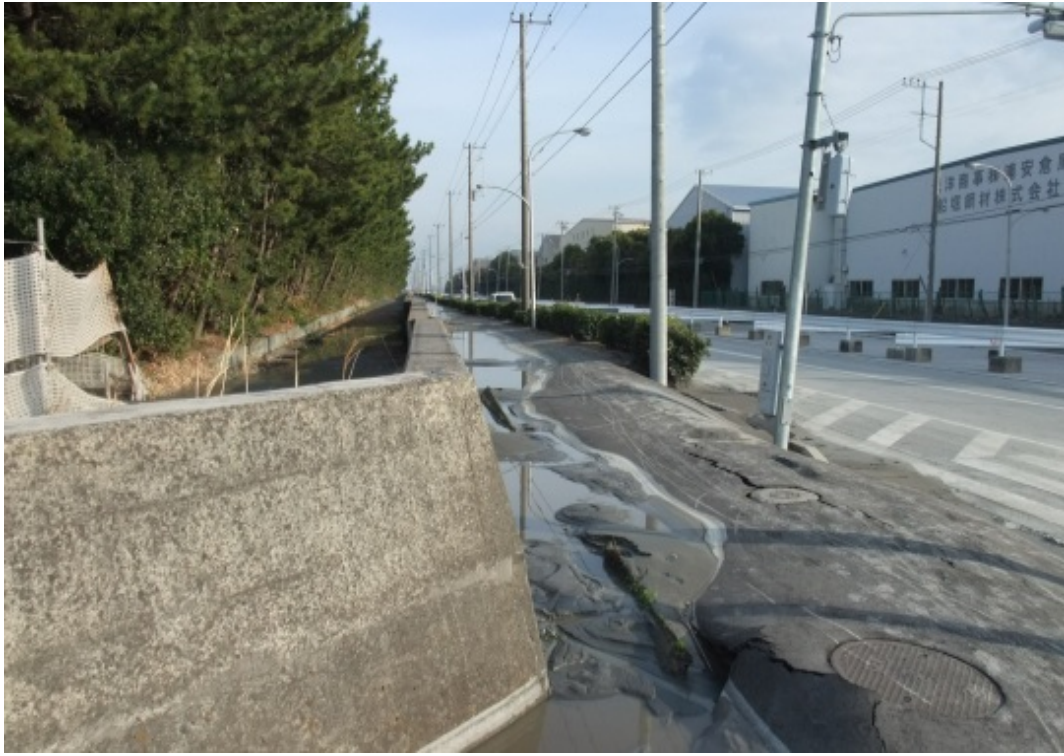
Photo 5 Heaving of a footway at Takasu in Urayasu City
