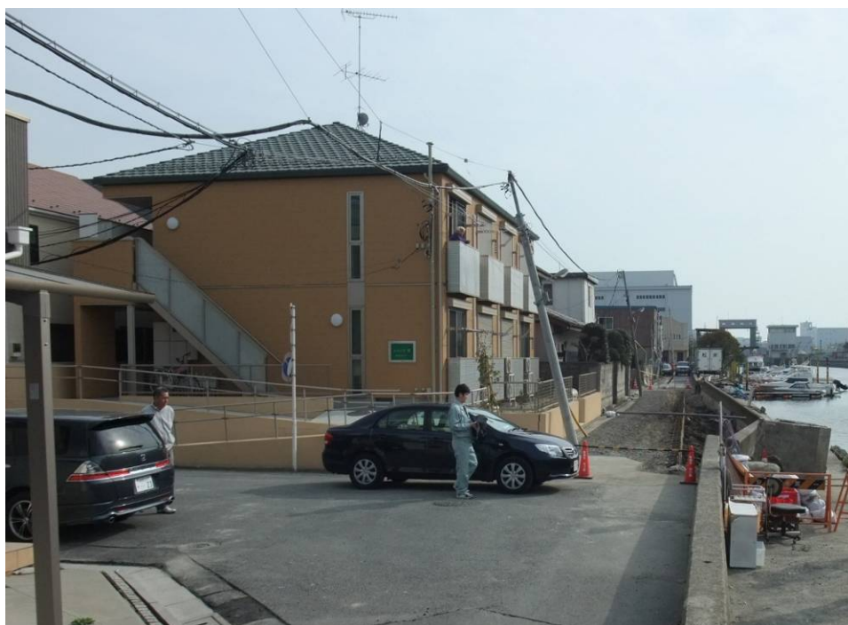
Photo 11 Tilted river wall in Funabashi City
