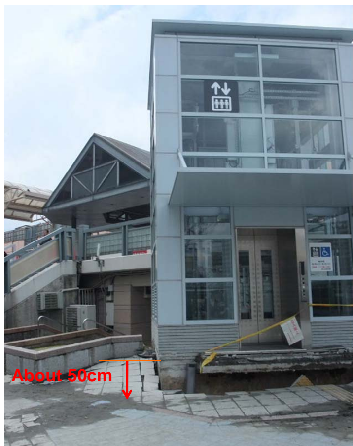
Photo 8 Large differential settlement in Shin-Urayasu Station
