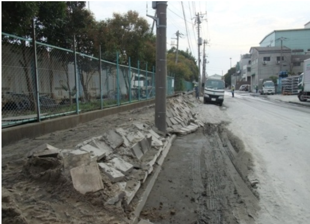
Photo 6 Heaving of a footway at Takahama in Ichikawa City
