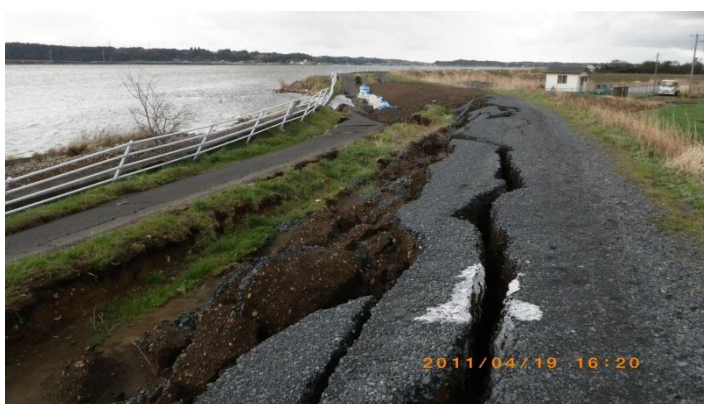
Photo 1. Liquefaction damage in Hinuma levee
