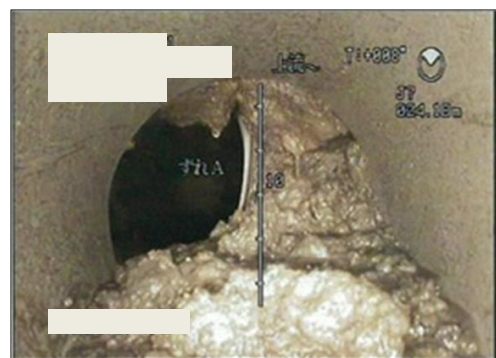
Photo 2. Disconnection of sewage pipeline and deposit of sand after liquefaction (damage study in Tokyo Bay area, 2011)
