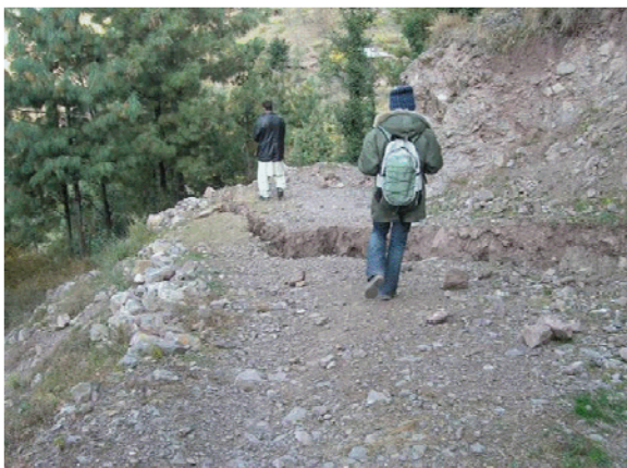
Fig. 1 Earthquake-induced crack in mountain slope (after the 2005 Kashmir earthquake).
