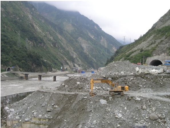
Fig. 7 Debris channel behind Beichuan City.
