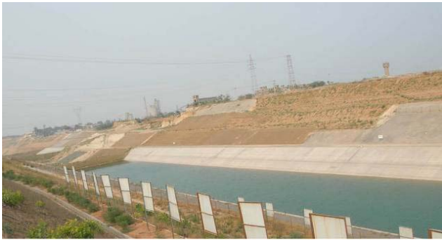
Figure 13 Part of Luwangfen test section in expansive soft rock (with courtesy of Professor Gong Bi-wei)
