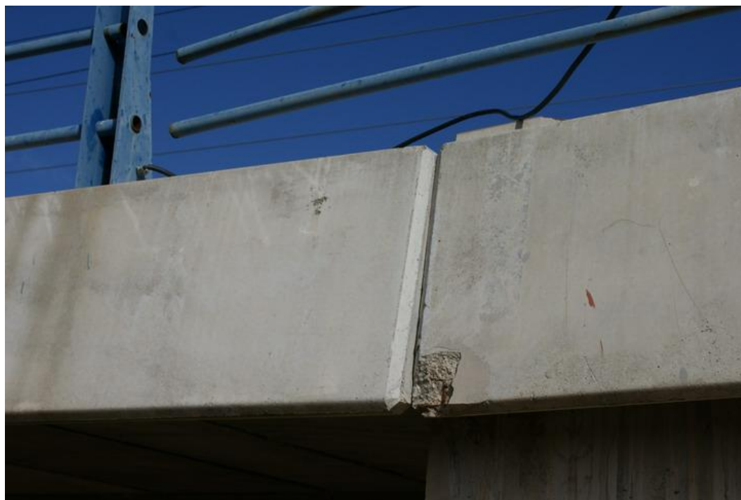
Damage in Pallaressos structure
