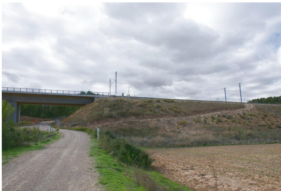
Pallaressos Viaduct and one of the access embankments affected by thaumasite crystal growth
