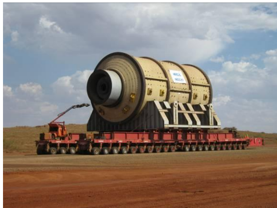
Tensar mechanical stabilisation of a temporary causeway over tidal mud flats, Australia
