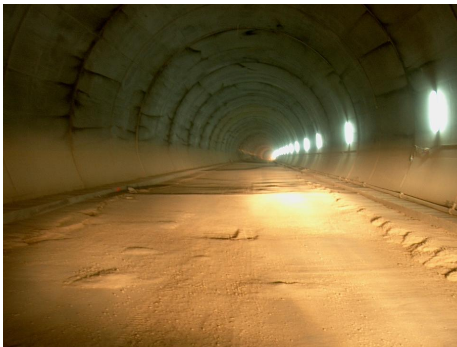
Lilla tunnel. Heave of the floor
