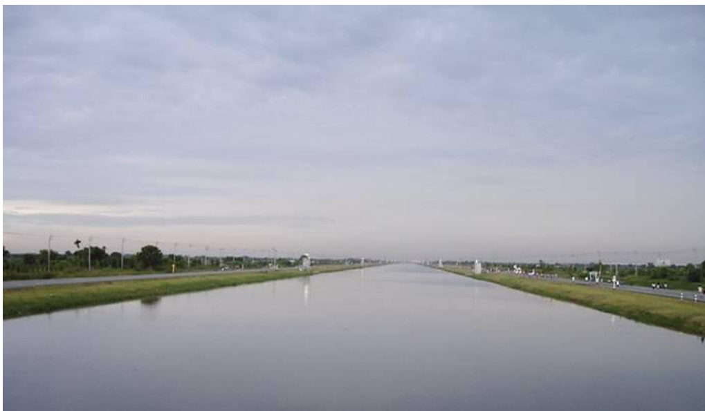
Fig. 4 Use of soil cement column in excavation of canal in the soft Bangkok clay, upper photo shows some related instability problem which had been solved and the lower photo shows the canal after completion
