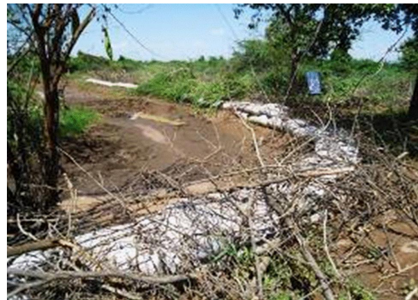
Figure 16 The dam's embankment built with “Do-nou” covered with the branches of Acacia
