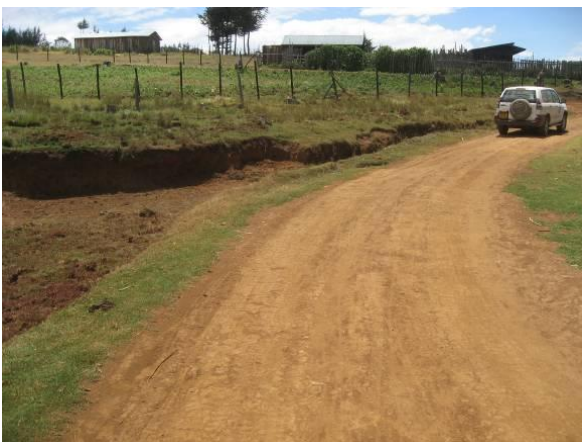
Figure 15 The road situation after two years of maintenance at the same place as in Figure 14 (Kenya)
