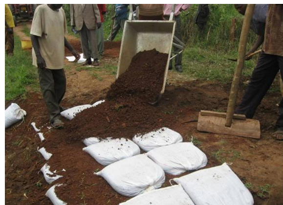
Figure 12 Gravel is distributed over the final layer of “Do-nou” to build the final layer of the road surface (Kenya)
