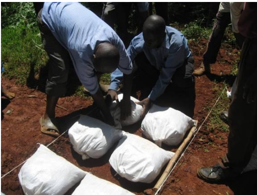
Figure 10 “Do-nou” are positioned at a site where the mud has been removed. The space between “Do-nou” is necessary to allow them to expand due to compaction (Kenya)
