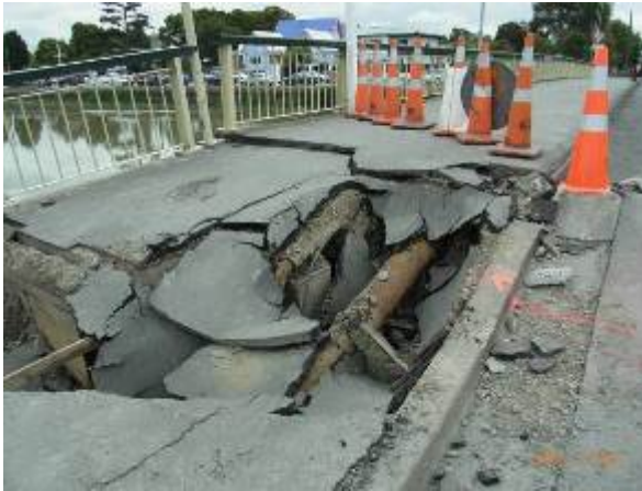
Photo 5 Pipeline damage at Avondale & Brighton on Avon River
