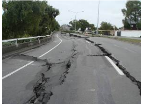
Photo 6 Collapsed portion of Fitzgerald Avenue
