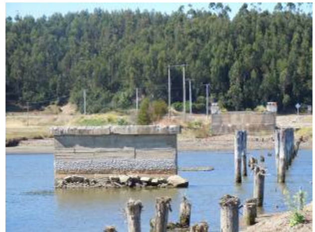
Subsidence of Tubul Bridge pier by 1 to 1.5 m because of subsoil liquefaction
