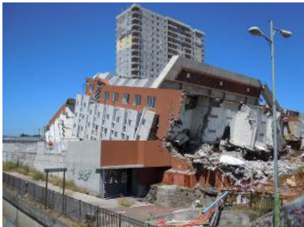
Collapsed building in Concepcion
