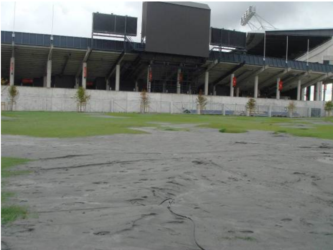
Photo 7 Liquefaction adjacent to AMI Stadium. The ground under the stadium was stabilized with stone columns. Around the stadium, liquefaction was observed everywhere, but the stadium did not suffer structural damage.
