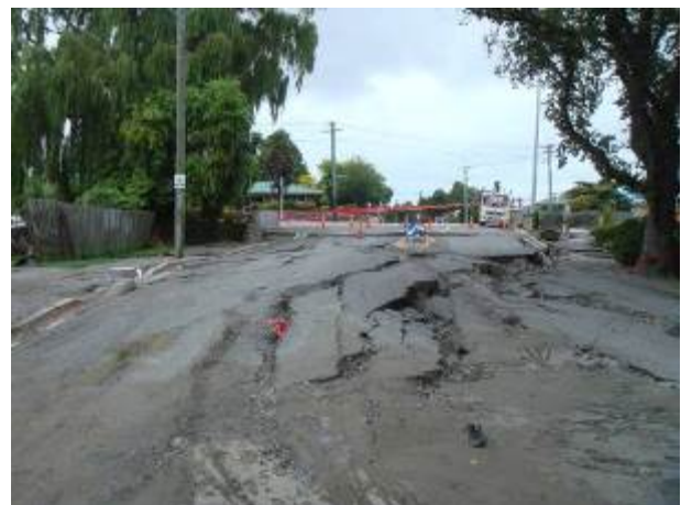
Photo 4 Damaged road embankment in Avonside Drive
