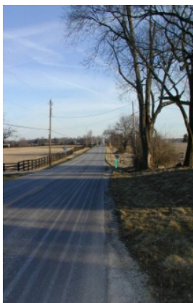
Figure1. Failing Delaware County Pavement
