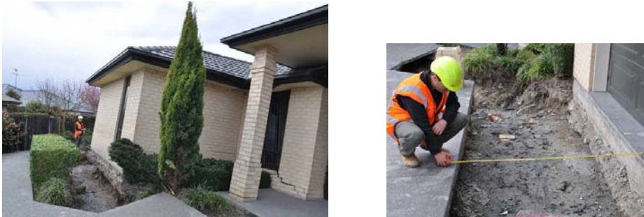
Figure 11. Severe damage to residential houses/properties due to lateral spreading in South Kaiapoi; (a) Excessive tilt and uplift of foundations due to lateral spreading; (b) The width of this crack increased from 1.4m to 1.6m in the period between 11 and 15 September (7-11 days after the mainshock).
