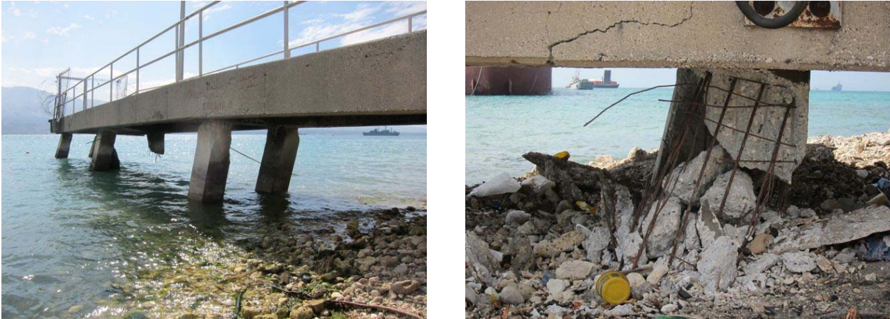
Figure 9 Damage to piles supporting the pedestrian bridge connecting the South Pier to the island
