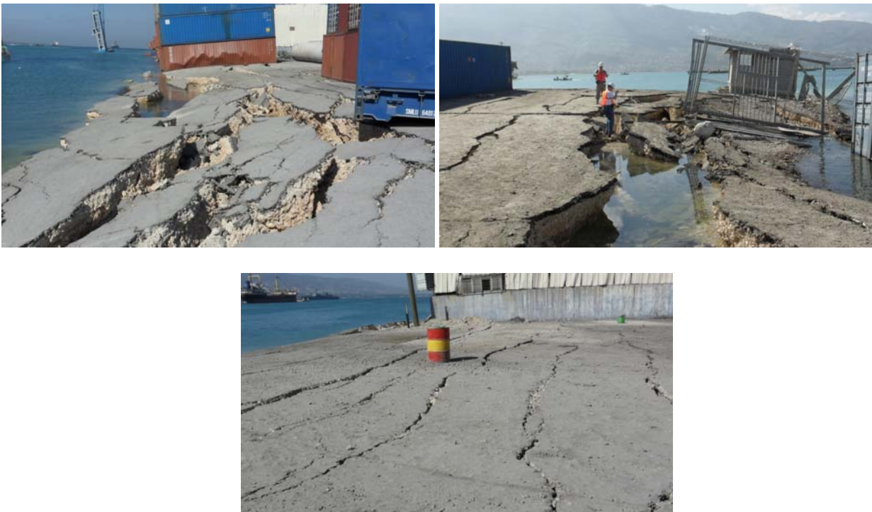
Figure 7 Lateral spread cracking and deformations along the North Wharf of the port.
