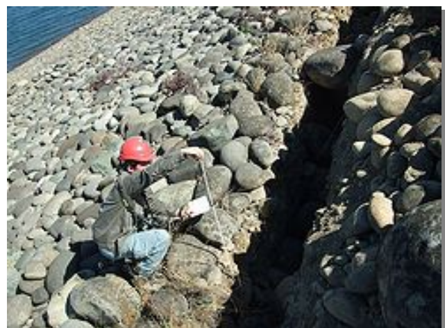
Photo 10 Downward slope movement in upstream face
