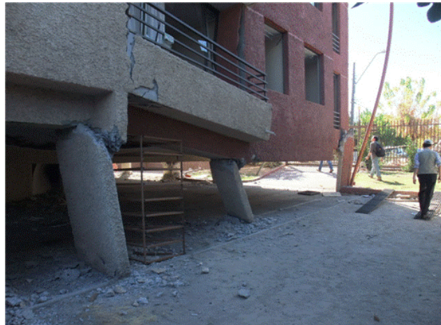
Photo 28 Collapsed building at Maipú in Santiago
