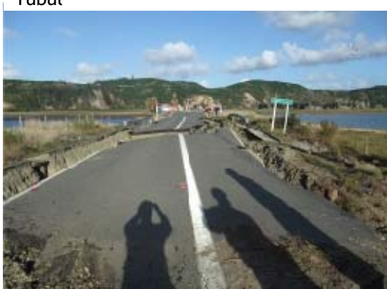
Photo 16 Collapsed approach embankment of Raqui II bridge
