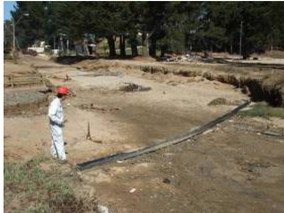
Photo 24 Exposure of buried lifeline after tsunami erosion
