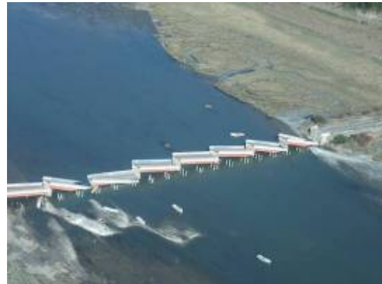
Photo 15 Collapsed bridge in Tubul
