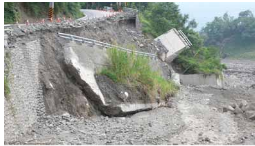
Figure 26. Erosion at bottom of retaining structure
