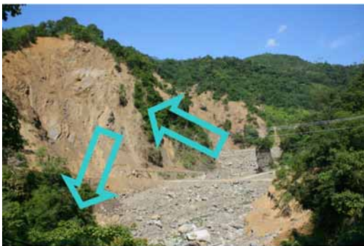
Figure 27. Erosion along curved river channel.
