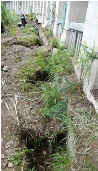
Figure 16. Subsidence in foundation of rock-shed tunnel
