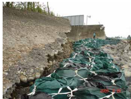
Figure 20. Erosion at toe of road embankment
