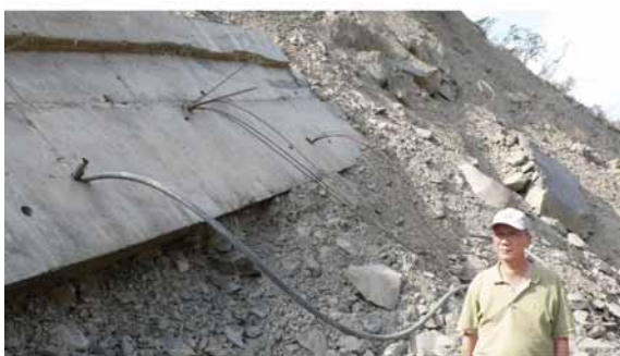
Figure 10. Destroyed shape of ground anchor.
