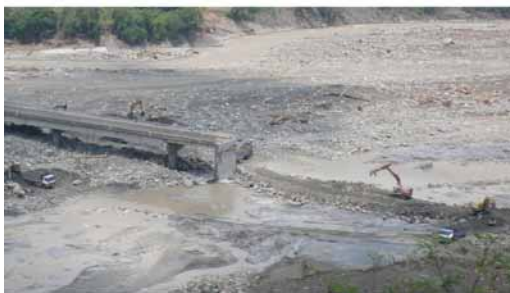
Figure 19. Bridge abutment and embankment destroyed by erosion
