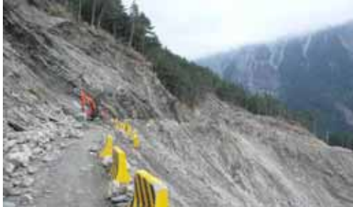
Figure 25. Big slope failure
