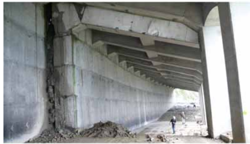
Figure 15. Distortion of rock-shed tunnel
