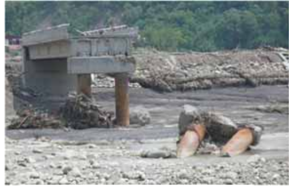
Figure 35. Scouring in bridge foundation
