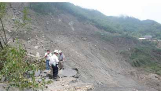
Figure 13. Mountain road destroyed by slope failure
