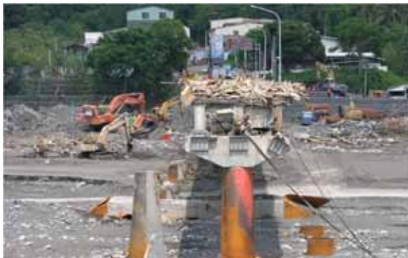
Figure 36. Accumulation of drifting wood on bridge deck
