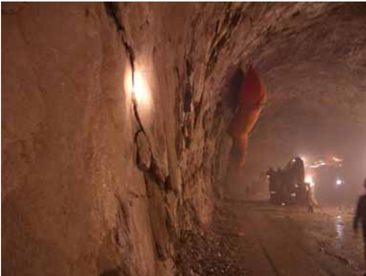
Figure 4. Rock spalling in the tunnel shoulder at the JinPing II hydroproject on the Yalong River, Sichuan Province, China.
