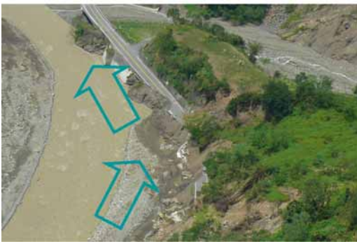
Figure 17. Toe erosion in river channel
