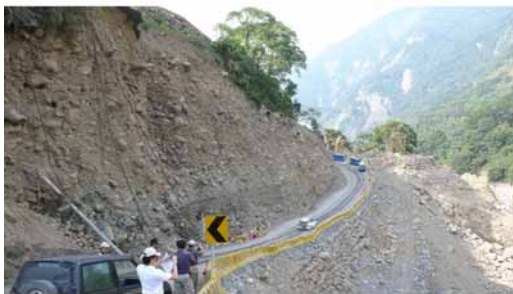
Figure 8. Failure of natural slope along road
