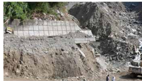
Figure 9. Collapse of retaining wall without stable foundation
