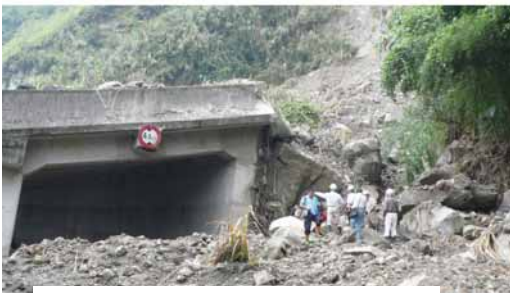
Figure 14. Rock shed tunnel subjected to slope failure
