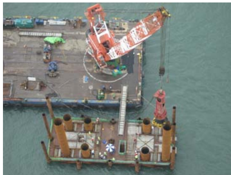
Figure 7. Driving the steel pipe pile of 1.8 m diameter using hydraulic hammer system
