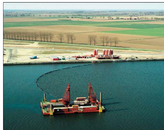
Figure 3b: The equipment for the stabilisation of the sludge
